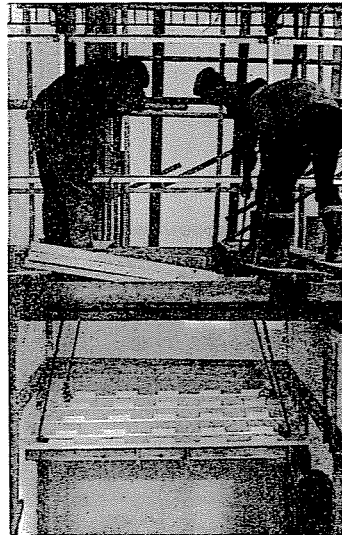
Photo 25. Erecting the test building gave an occasion to experiment with a novel technology; creating the first horizontal load-bearing tissue-structure by in-situ pouring. For this purpose a light auxiliary timber grid has been constructed on top of which the floor element was placed. Four holes were drilled into the gypsum and thereby the ropes — ending in screws — could be directly fastened to heterogeneous jointing points built into the timber grid. When the floor unit was lifted into position, little auxiliary beams were fastened underneath, to jointing points embedded into the reinforced concrete beams. In this case reinforcement is directly placed into the open two-way channels from above
